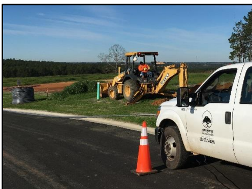
Terry Gantt working a job in Aiken, SC installing electrical conduit for the client in a new subdivision.
